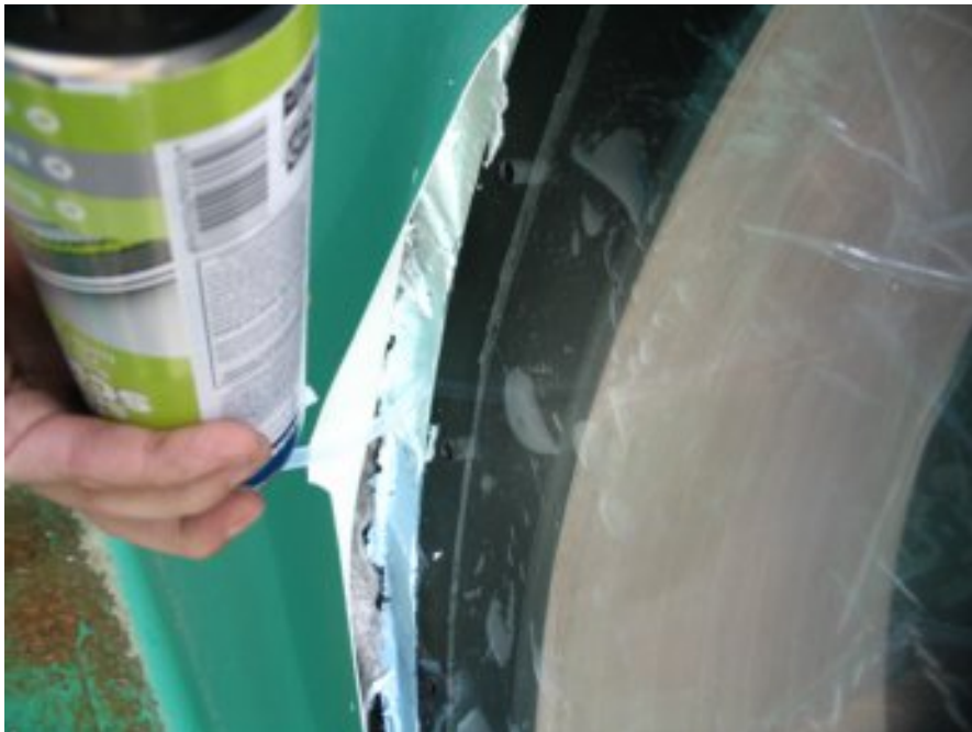
Abbildung 8: The space besides the window block is filled with 2 component polyurethane foam
