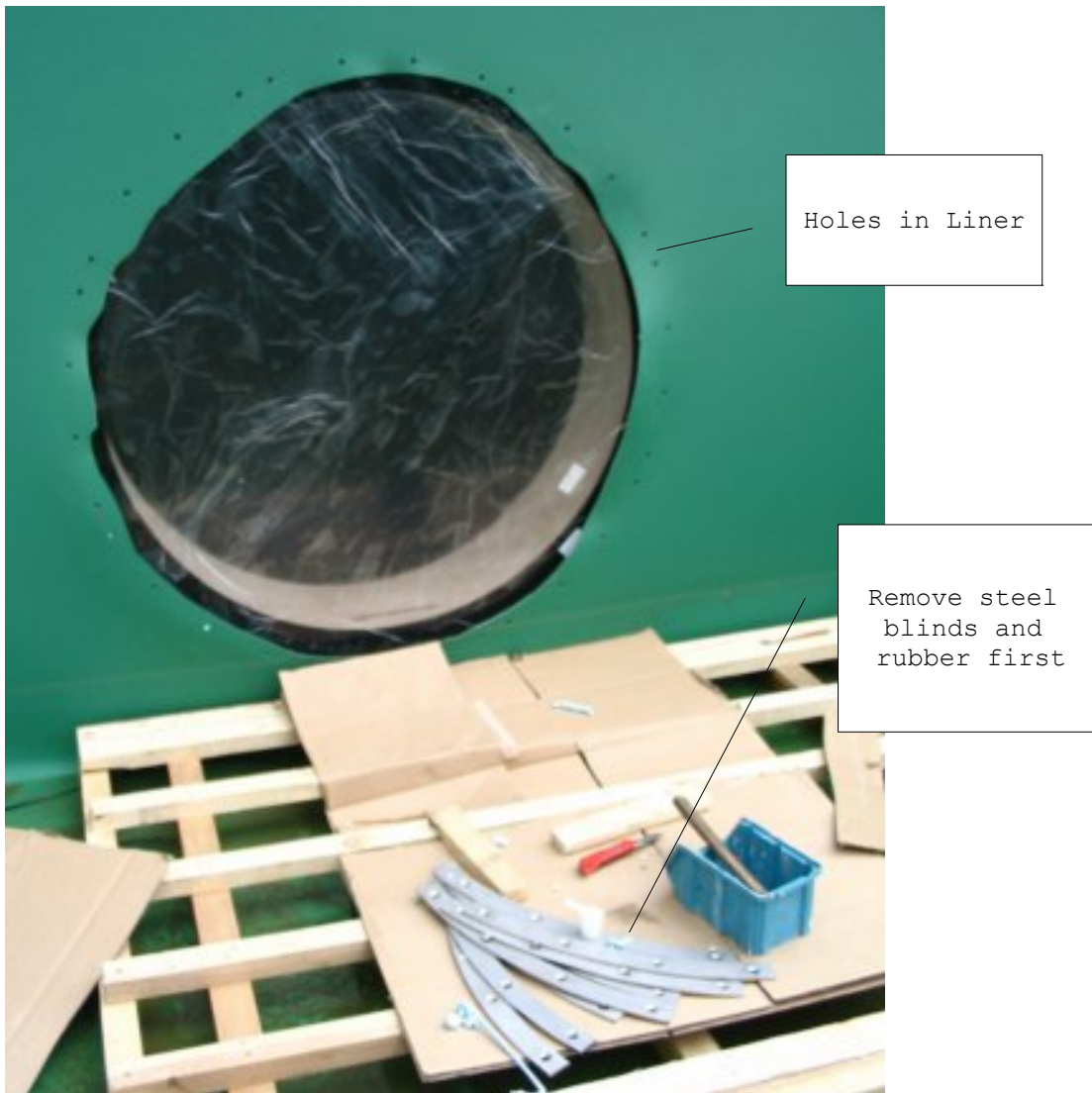
Abbildung 10: Make holes in (green) liner with a power drill – using a large steel drill. Cut remaining parts with sharp cutter knife.
